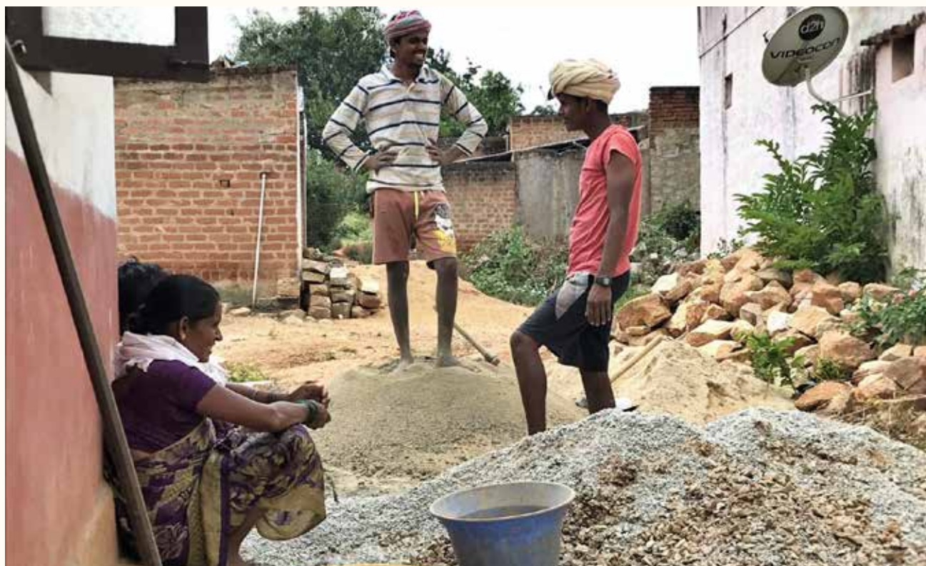
Nanda and Anil with their mother during a construction activity (Photo: Saumya)
